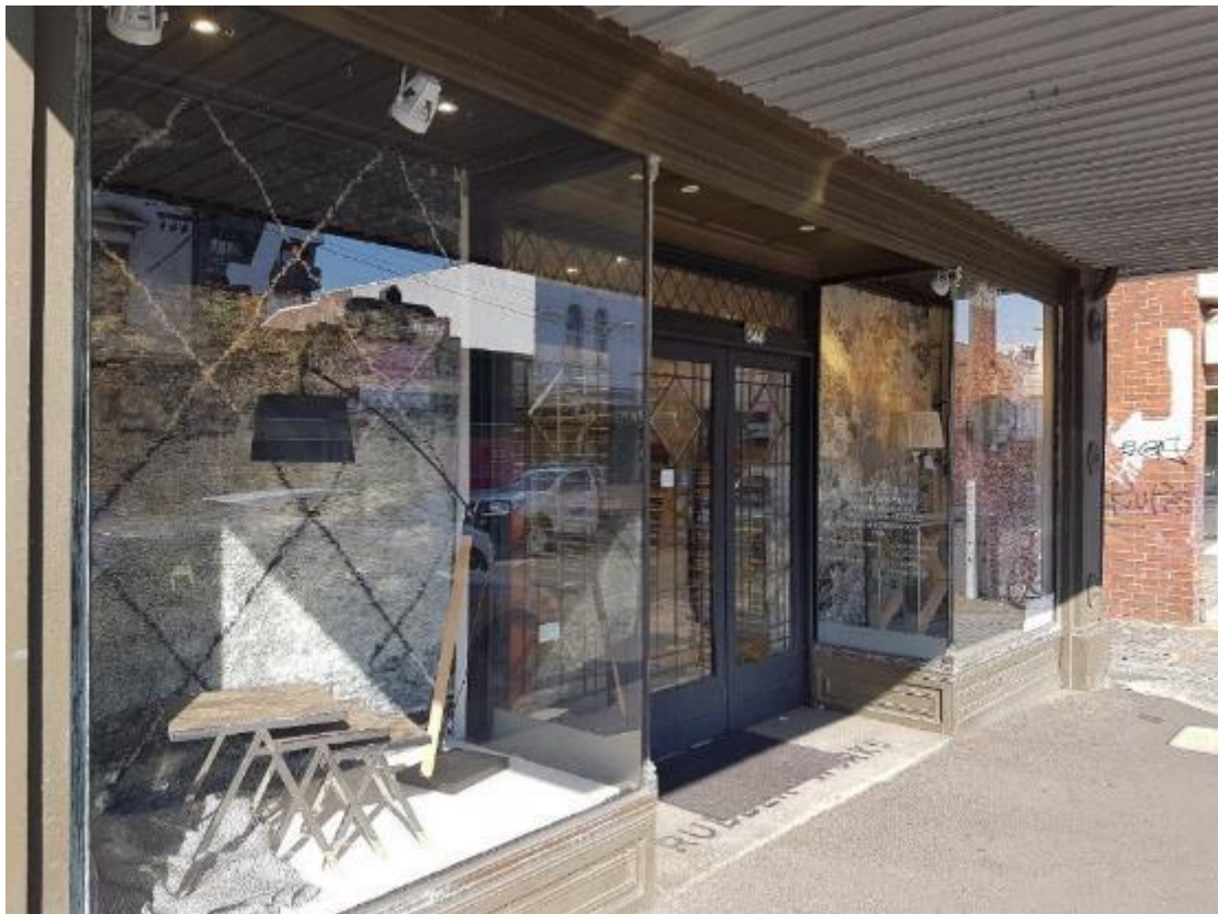
Figure 5. Intact shopfront comprising ingo with 'Lion Rubber Works' imprint, Greek Revival doorway, metal framed windows and timber stalls. (Source: Trethowan 2017)
