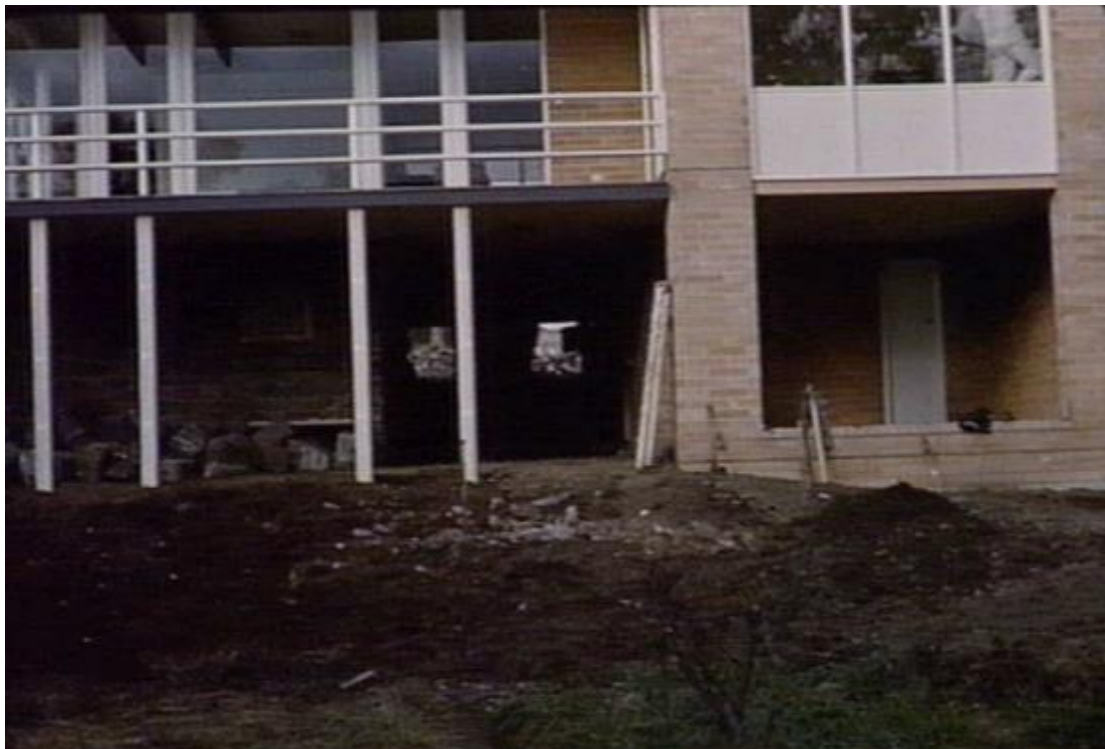
Figure 1. View of the lower-ground floor of the house, during construction, from the rear garden. (Source: State Library of Victoria)
