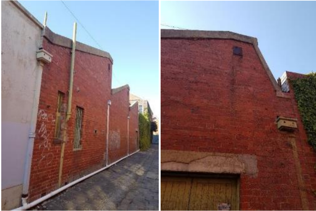
Figure 8. View of factory section and detail of roof end over alley doorway. (Source: Trethowan Architecture 2017)
