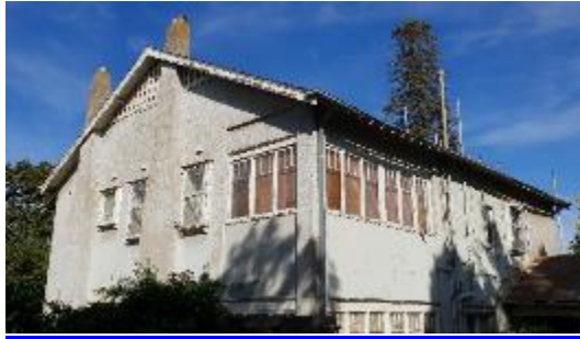
Figure 7. Northeast corner of the house showing infilled rear balcony. Source: Trethowan Architecture 2019
