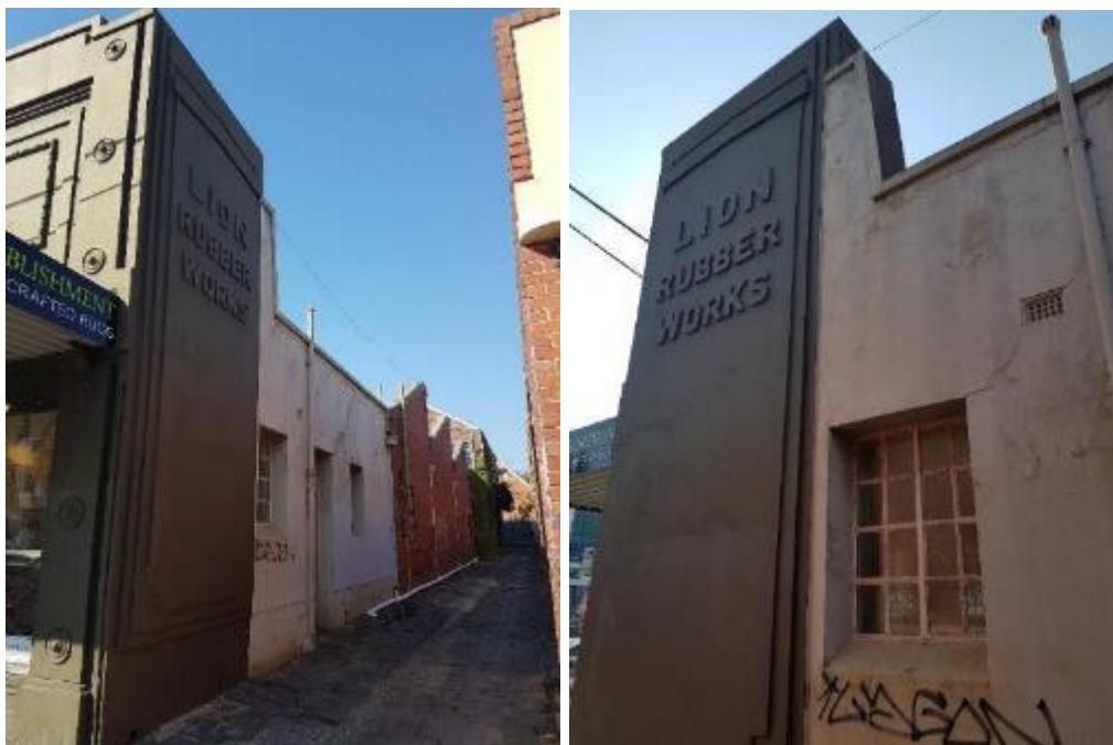
Figure 7. Signage on west façade and view into alley showing shop and factory sections of the site. Close up view of side window with wire glass in steel frames. (Source: Trethowan Architecture 2017)
