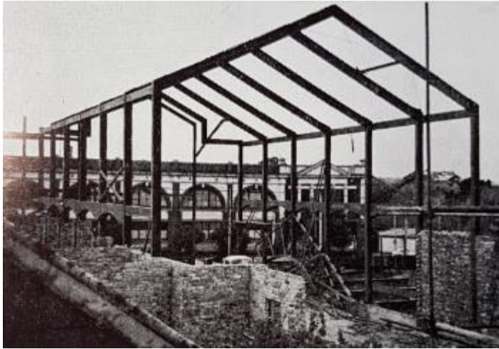
Figure 8. Erection of the steel frame of the basilica. (Source: Santuario di S. Antonio 1969)
