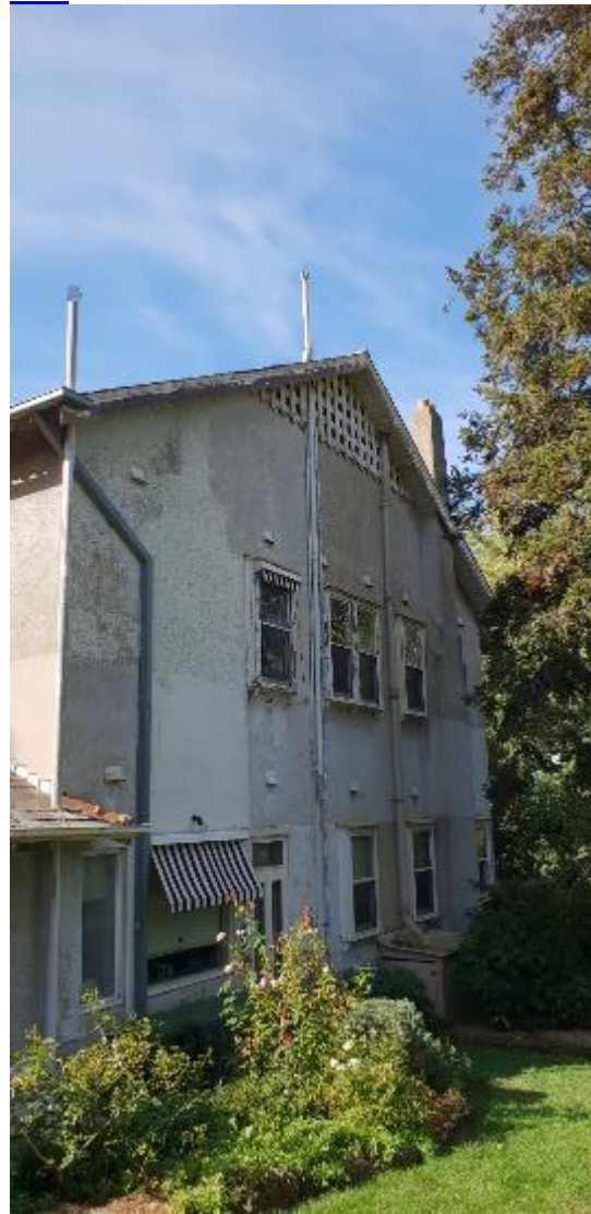
Figure 10. View of the western elevation showing intact chimney, are where chimney has been removed, intact box windows, rendered wall and timbered gable end. Source: Trethowan Architecture 2019
