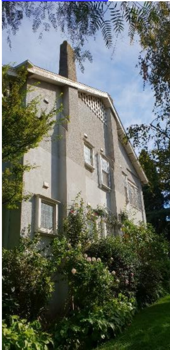
Figure 9. View of the eastern elevation showing rough render and smooth band, intact chimneys, box windows and timbered gable ends. Source: Trethowan Architecture 2019
